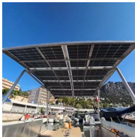
Solar canopy 1600 Wp
