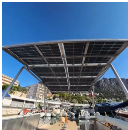
Solar canopy 1600 Wp
